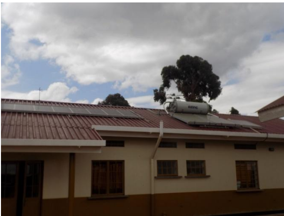
Martenate Ward with Solar at Mwizi HCIV
