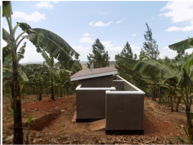
2 Stance VIP Latrine at Rwinyaga P/S in Mwizi S/C
