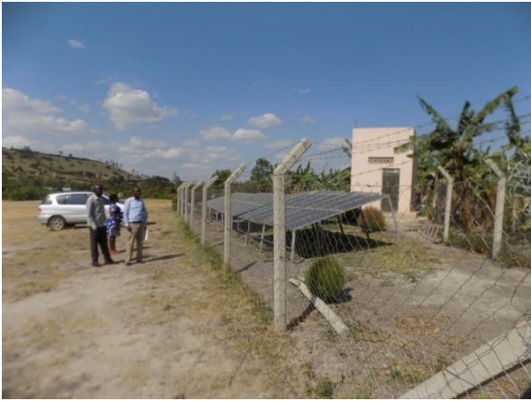
Solar Powered water system in Rubaya S/C
